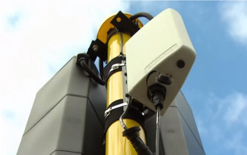
Figure 9: ITS-G5 Road Side Unit attached to traffic light.
