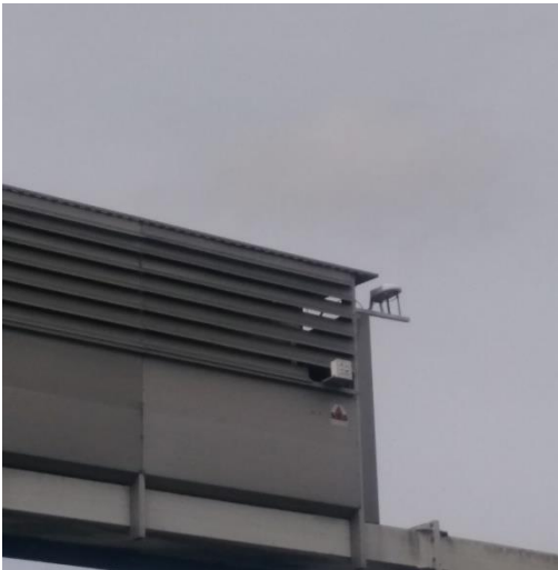
Road side unit on a VMS in Vendeville (A1)
