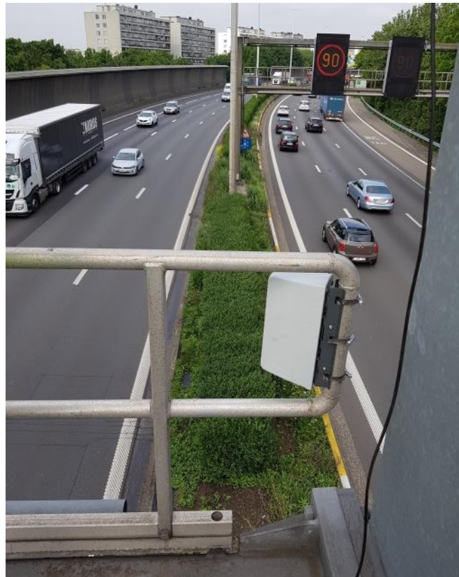
Figure 16: RSU mounted on gantry on E313
