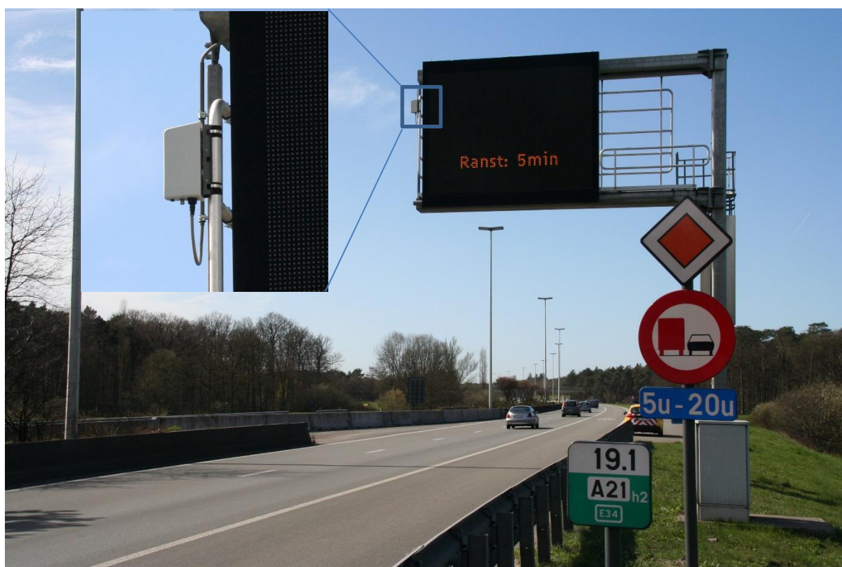
Figure 14: RSU mounted on gantry on E34
