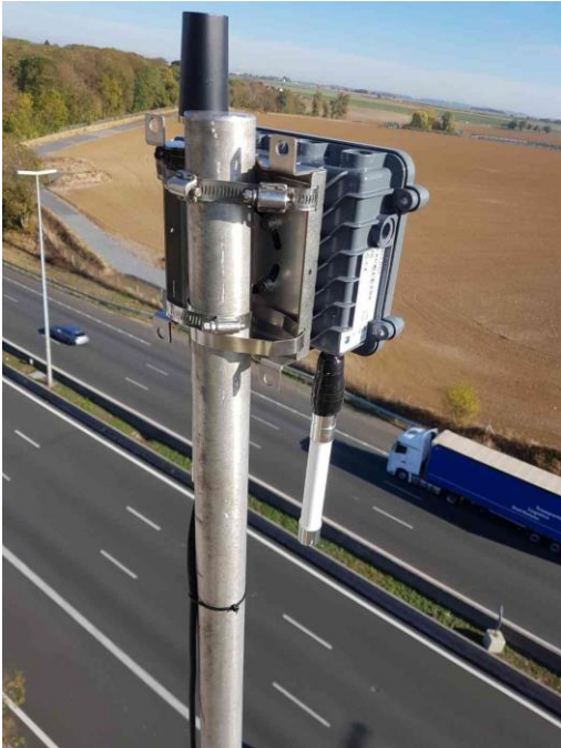
Road side unit on a pylon in Chennevieres-les-Louvres (A1)
