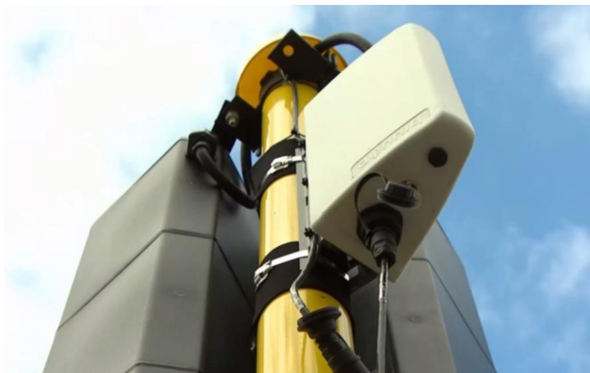
Figure 10: ITS-G5 Road Side Unit attached to traffic light.
