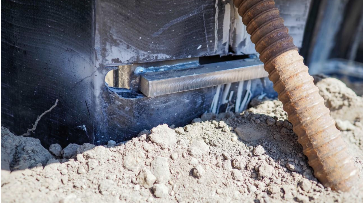
Figure 9-5 Local buckling and delamination of the outer 0/90 laminate layer
