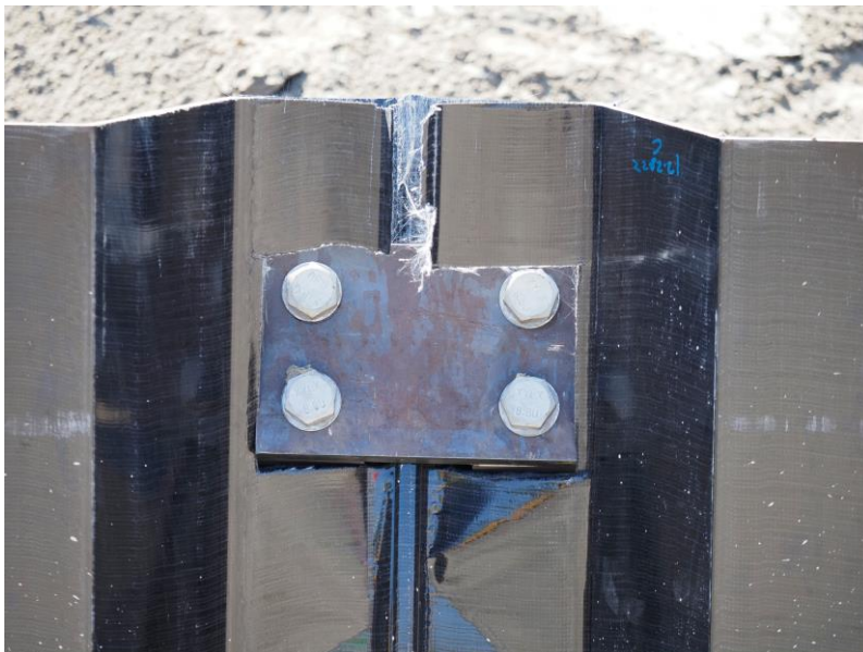
Figure 9-1 Punching shear connection plate and delamination
