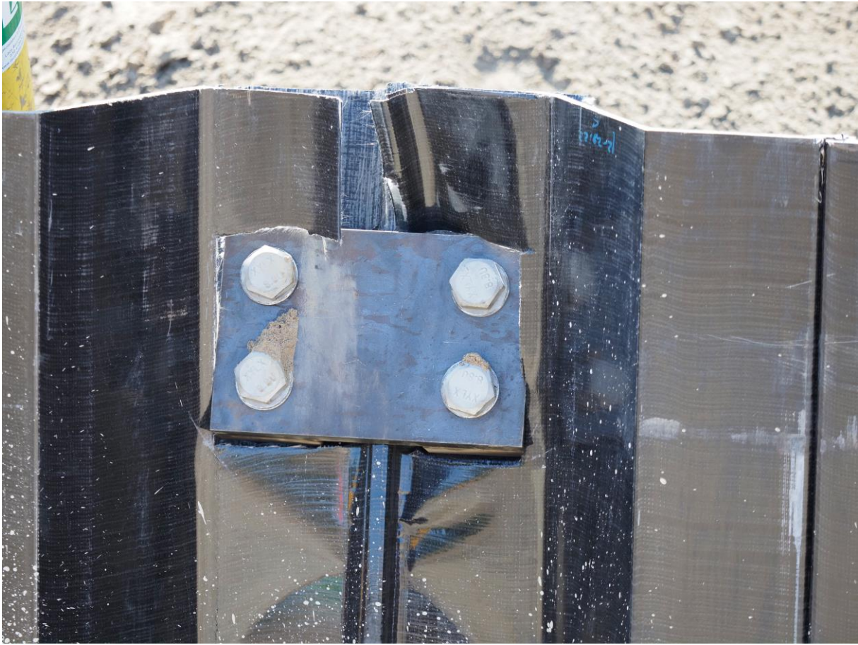
Figure 9-2 Punching shear connection plate and delamination
