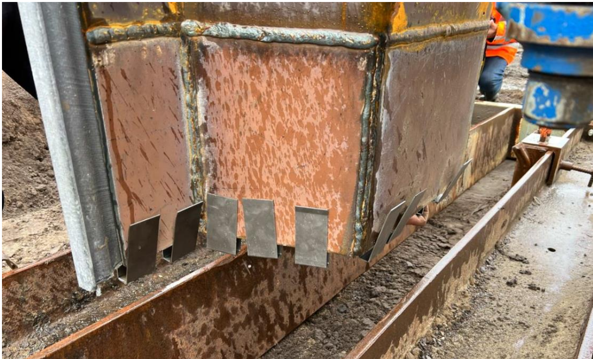
Figure 5-1 Auxiliary sheet pile with clips
