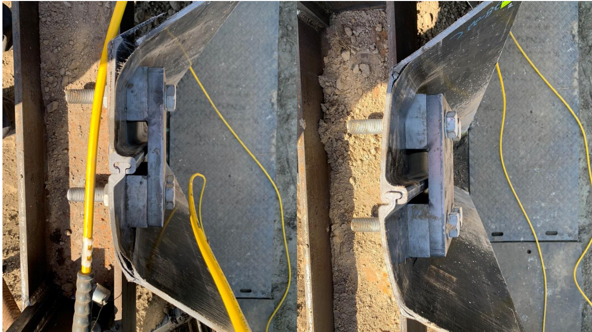
Figure 9-3 Punching shear connection plate and delamination
