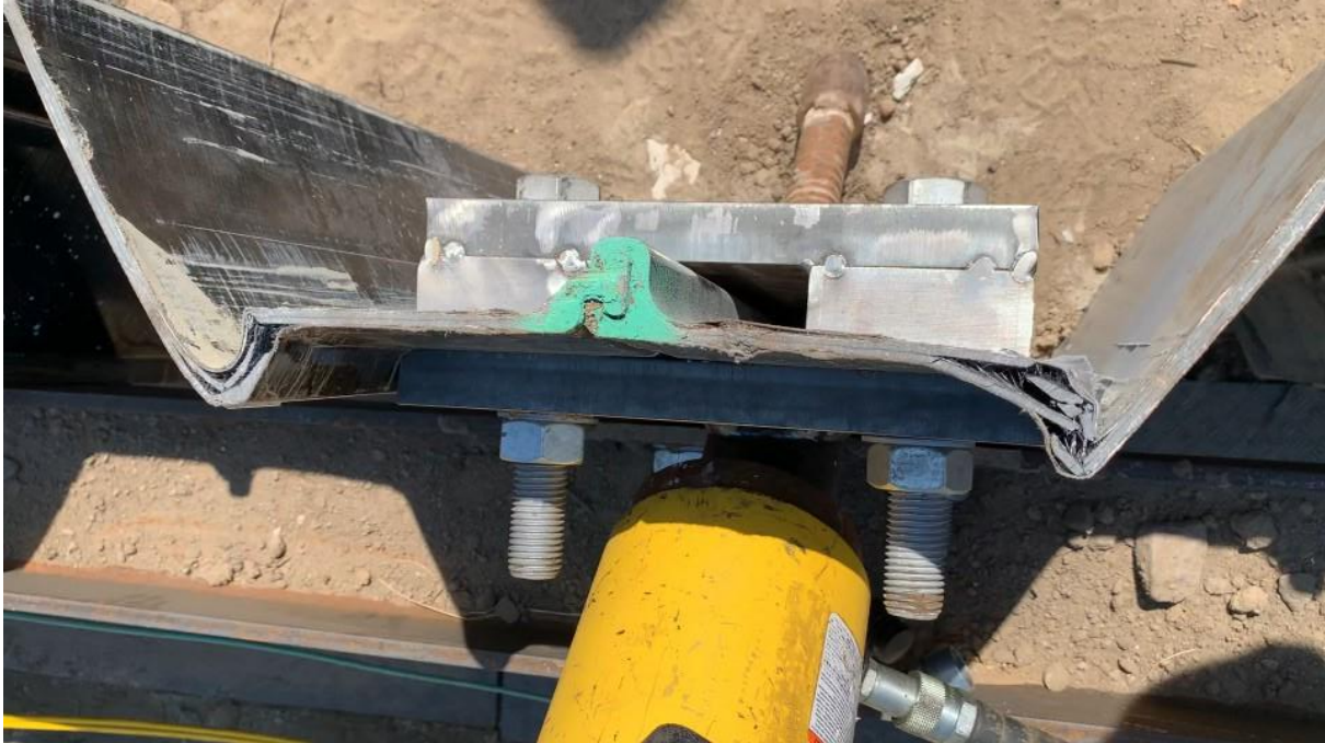
Figure 9-11 Local buckling and delamination of the outer 0/90 laminate layer
