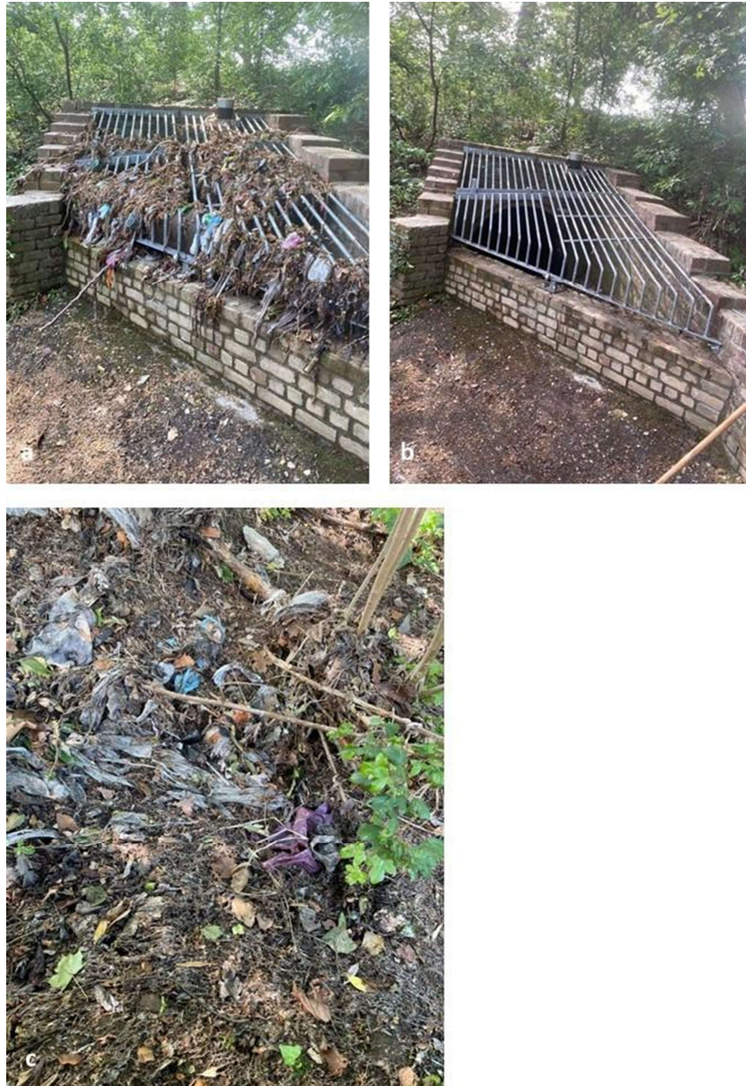
Figure 17. Overflow Gebroeders Koenraad park in Nijmegen. a) The overflow end after an overflow; b) the overflow end after cleaning; c) waste that remains in the park after an overflow event.
