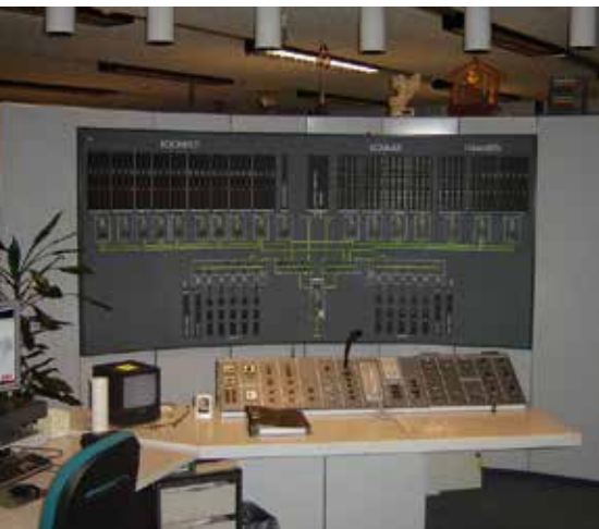
The operation panel in the control room of the ir. J.W. Topshuis
